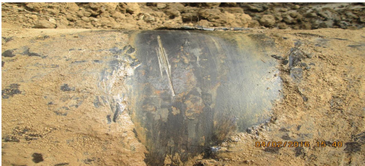
Fig 4: Spill point (Hack saw cut)
